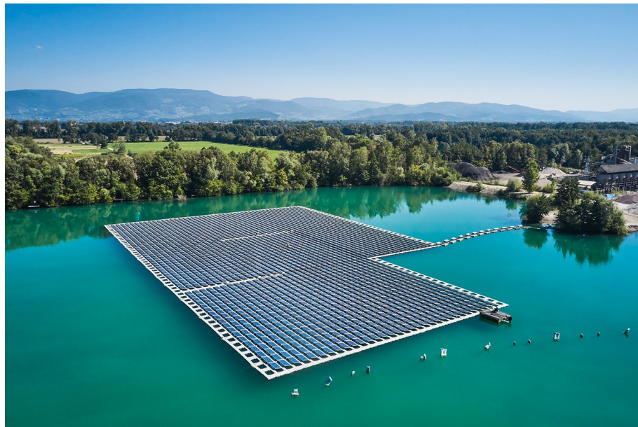
Figure 1. Floating PV power plant installed on Lake Maiwald with a net capacity of 749 kWp near Renchen/Baden. Photo: Jan Oelker.
